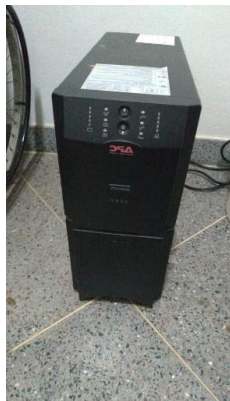
xiv. NOBREAK SMART-UPS 3000
